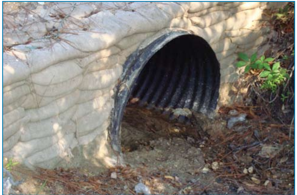
Figure 3.2-4. Culvert with sandbagged headwall is being used in a sandy soil drainage ditch. This method should not be used for permanent use in water courses.
