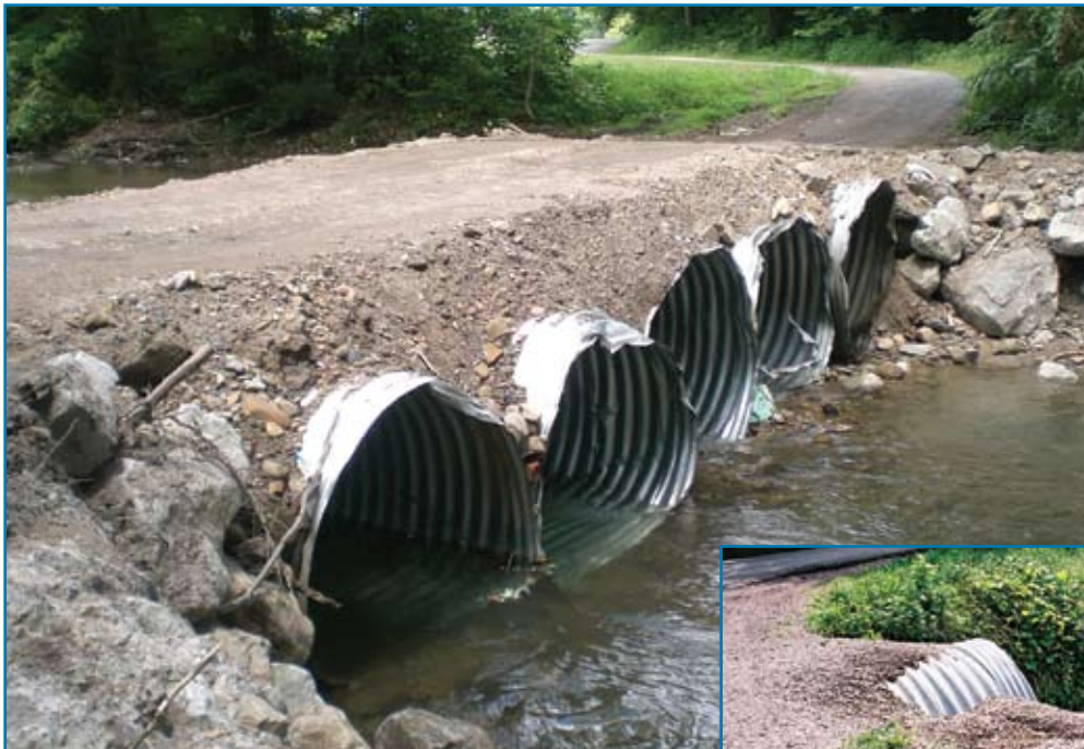
Figure 3.2-2. This multiple culvert crossing is vulnerable to debris blockage and washout. To install multiple or a “gang” of culverts properly, each culvert must be spaced adequately to allow for proper soil compaction between the culverts. This fill must be well armored at each end to prevent the washing out between the culverts.
