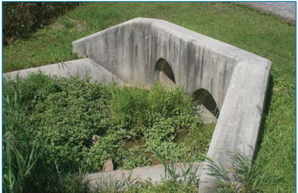
Figure 3.2-5. Multiple culverts at driveway ditch crossing have adequate spacing and compaction. The concrete headwall and wing walls help direct water flow and prevent washouts during high water flow. There is also adequate cover and culvert length to allow liberal clearance of traffic.
