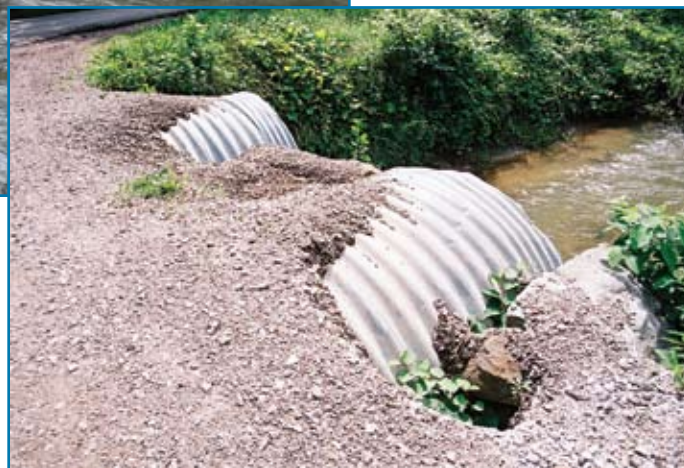
Figure 3.2-3. (right) Insufficient cover for culverts will result in washout and erosion as well as structural failure and collapse of culverts.
