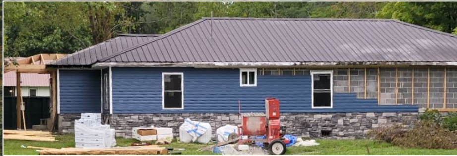
Substantially Damaged Structure Repaired
